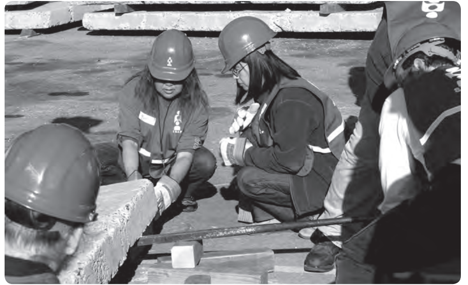
SNAP participants learn how to lift and move heavy debris like this concrete slab
